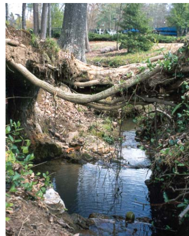
Figure 1. Excessive stormwater results in erosional damage to stream channels.
